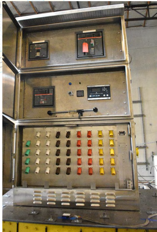
UUT-09 interior view.
