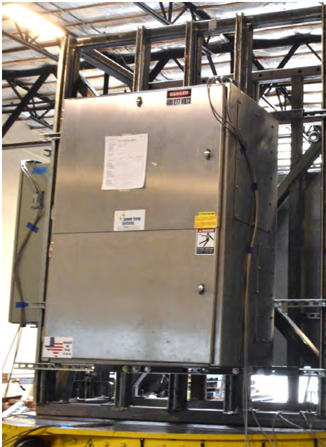
Over all view of UUT-06.
