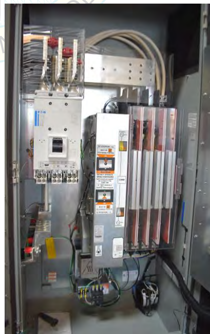
UUT-05 interior picture
