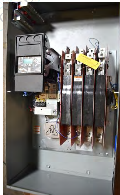
UUT-01 interior picture
