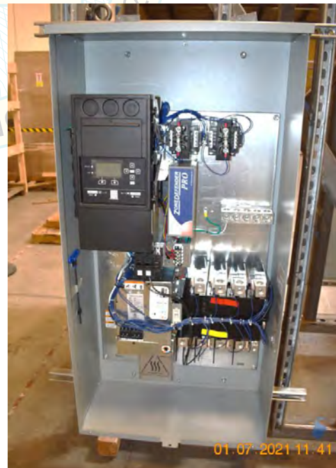
UUT-06 interior picture
