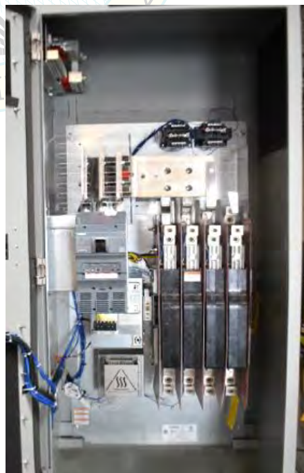
UUT-04 interior picture
