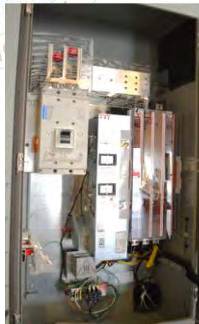
UUT-03 interior picture
