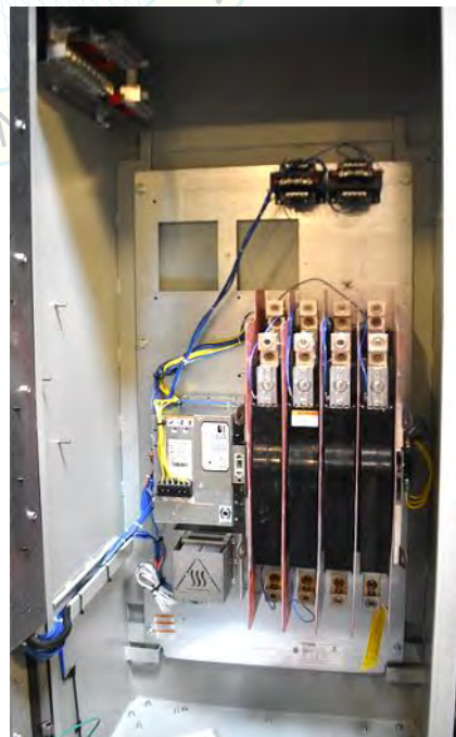
UUT-02 interior picture
