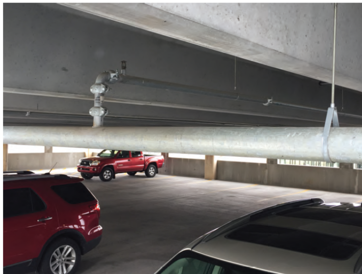
Sprinklered open parking garage.
