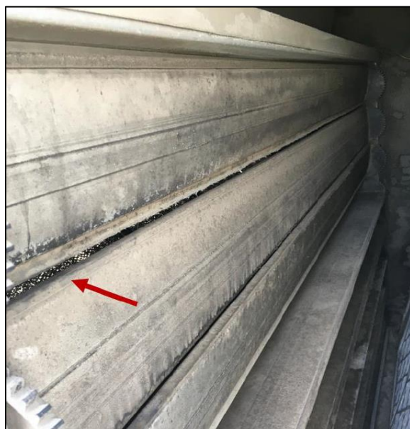
Figure 7.5 – Warped Damper Blade Unable to Close
