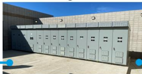
12kV Microgrid Gear
