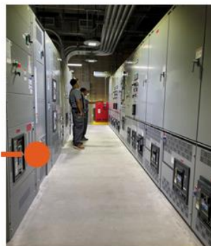
12kV Paralleling Gear
