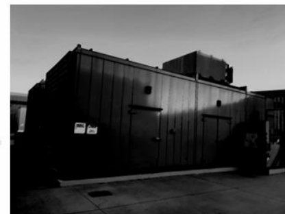
12kV Emergency Generators
