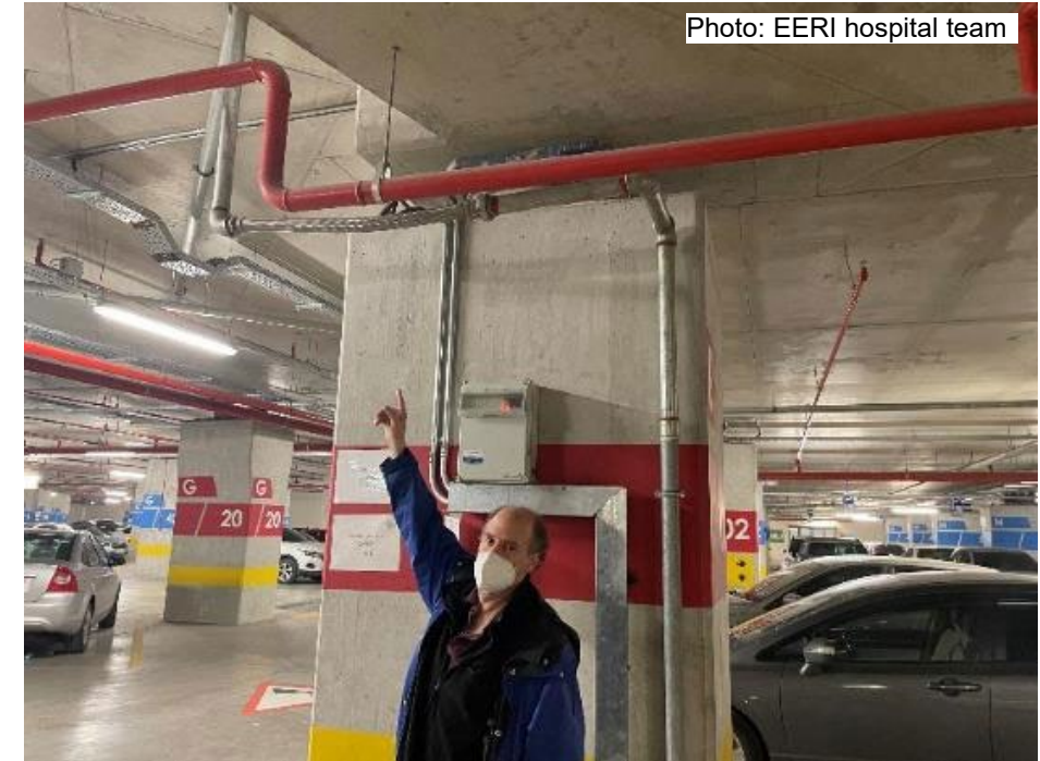
Adana City Hospital Flex connection provided for piping but does not have axial extension capability for isolator movement
