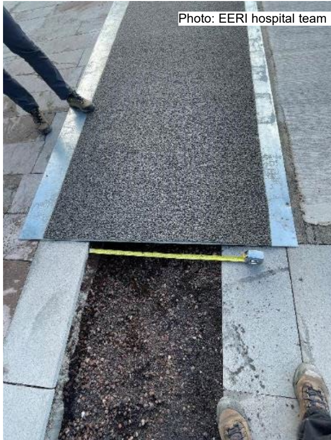
Osmaniye Government Hospital Moat gap filled with gravel
