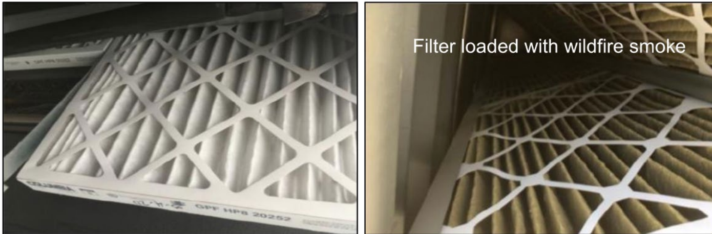
Figure 7.3 – Filter Before and After Load From Wildfire
