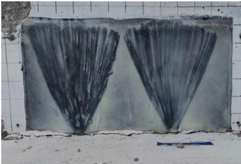
c. Shear failure at connection - SP11
