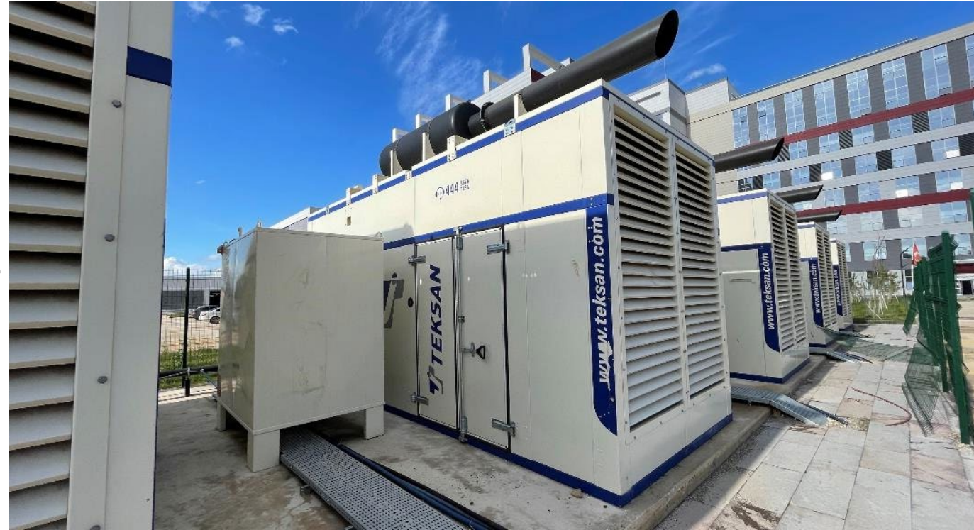
Osmaniye Government Hospital Emergency generator farm
