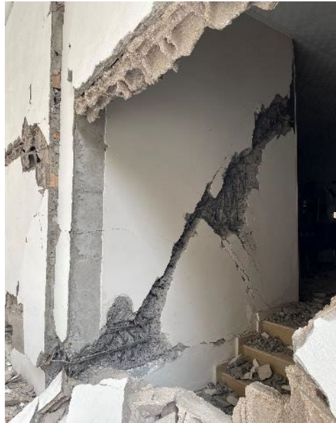
Shear Wall Damage
