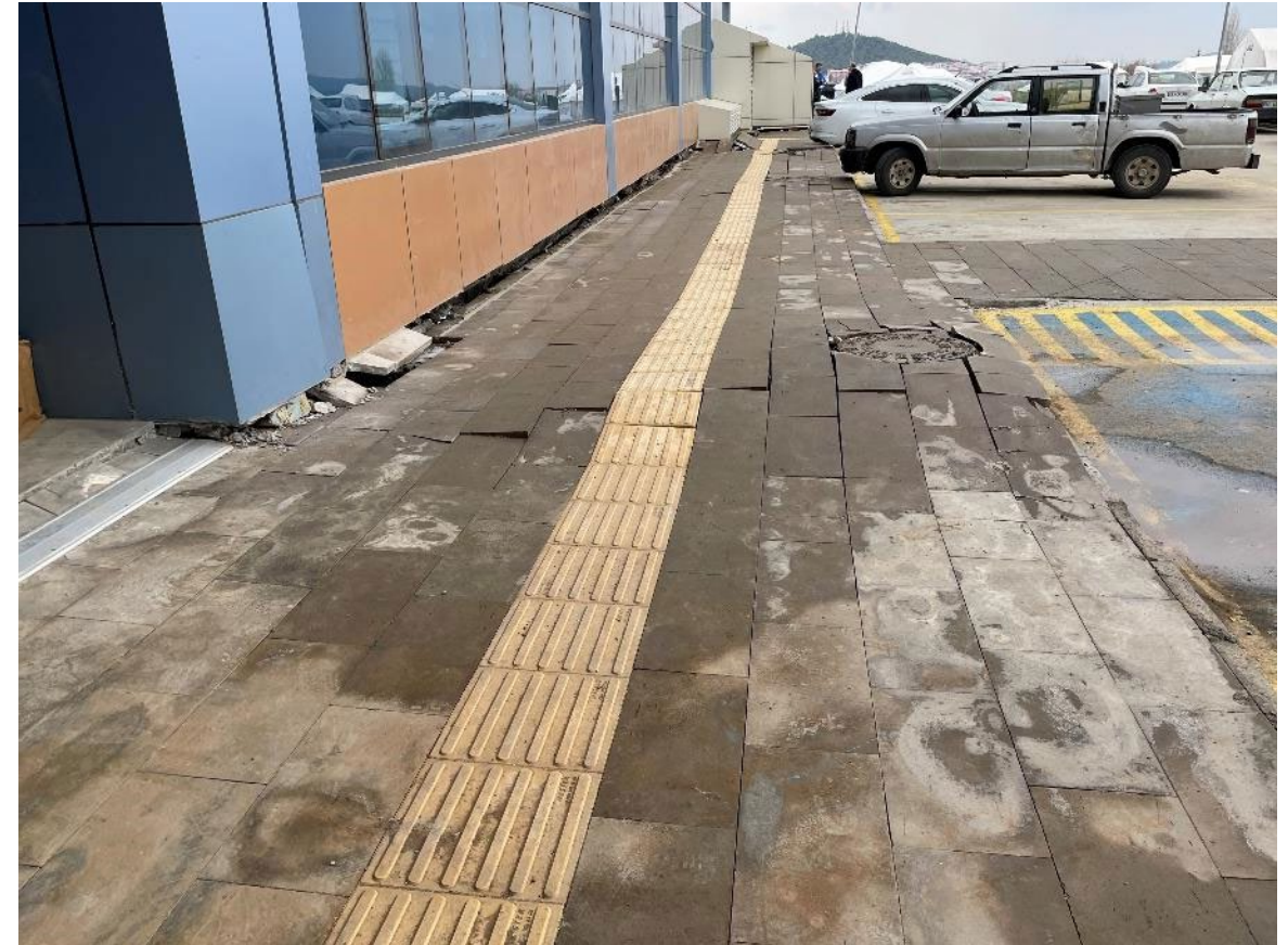
Pazarcik Government Hospital Soil settlement around perimeter of pile-supported hospital
