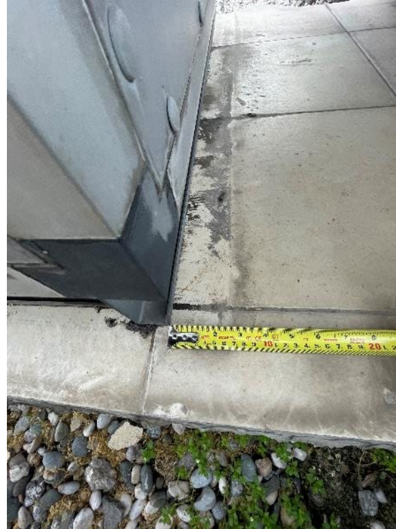
Markasi Hospital Kahranmanmaras Unanchored roof fan slides on pad
