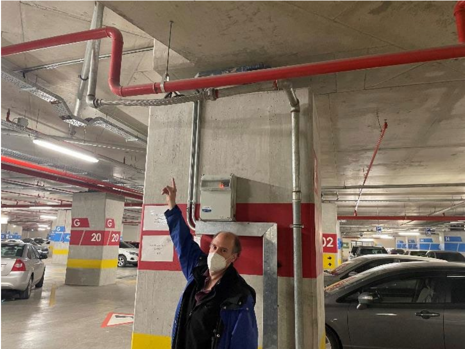
Adana City Hospital Flex connection provided for piping but does not have axial extension capability for isolator movement
