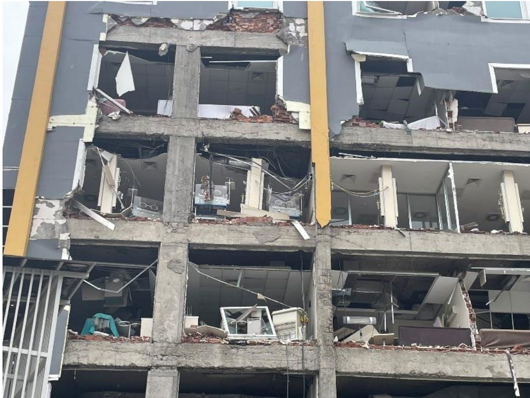
Megapark Hospital in Kahramanmaraş Infill damage and poor concrete frame quality, but no significant frame damage visible
