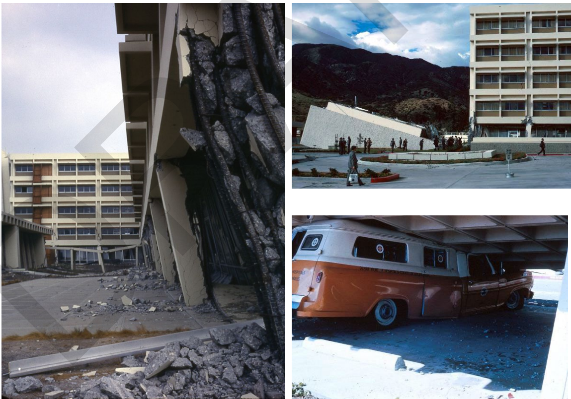
Figure 4. Damage to the Olive View Hospital during the 1971 San Fernando earthquake 4
