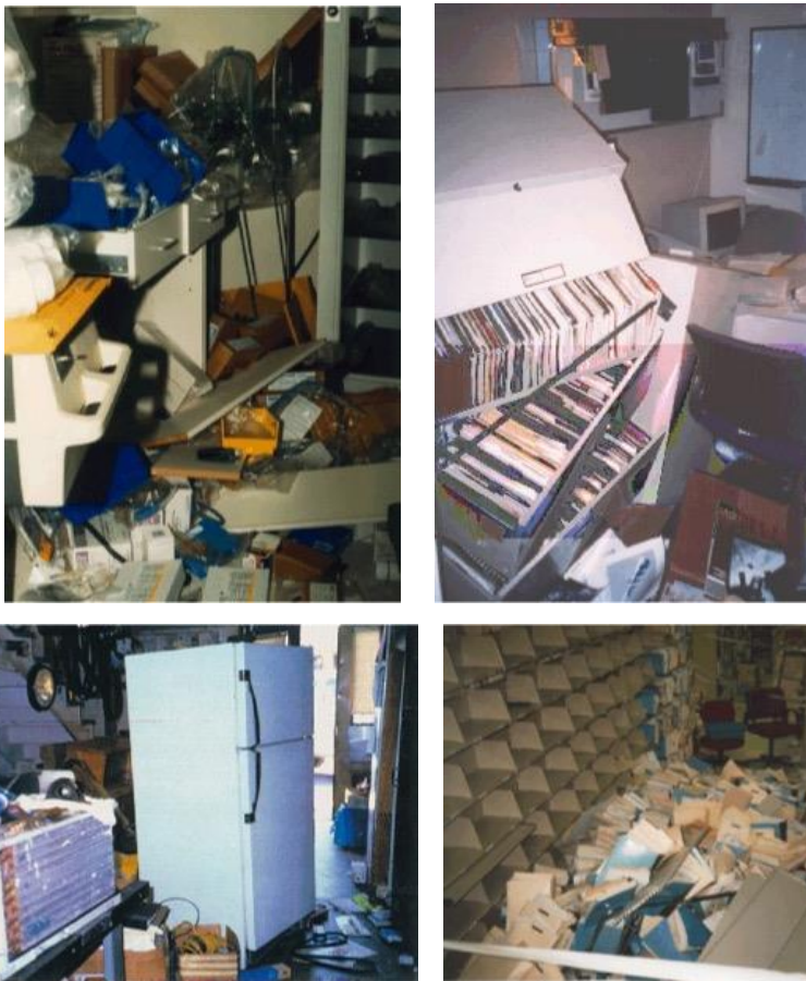
Figure 11. Examples of nonstructural damage at the new Sylmar County Hospital during the 1994 Northridge earthquake 10 .
