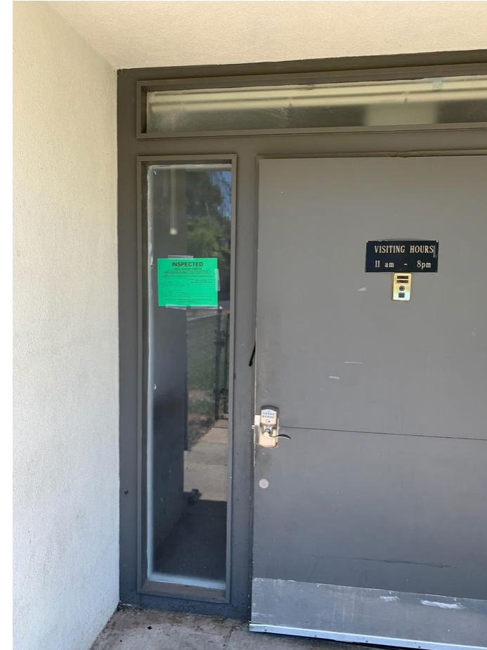
20015 - Feather River Care Center Cleared for repopulation by HCAI field staff and CDPH 7/5/2024
