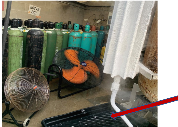
Figure 5 Provide Water and Spill Containment Below Evaporator
