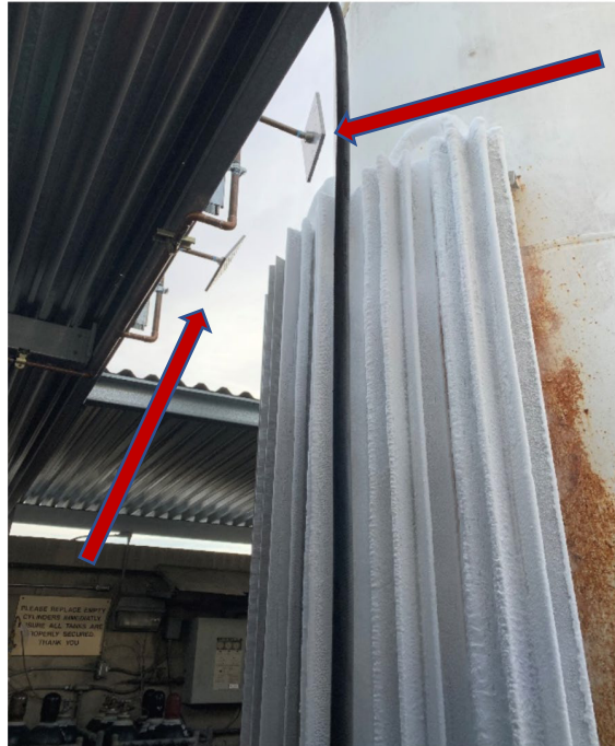
Figure 2 Sprinklers Used for Deicing
