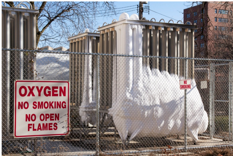
Figure 1 Ice on Oxygen Evaporator Piping
