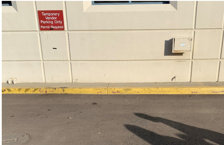
Figure 9 Emergency Liquid Oxygen Connections Shall Not Be Over Asphalt
