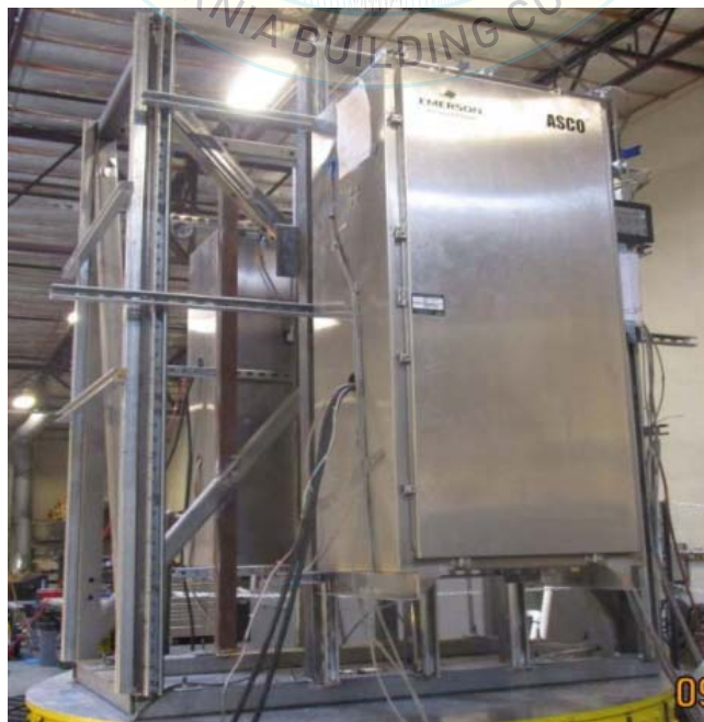
All units were filled with contents and maintained structural integrity and functionality after AC-156 test.
