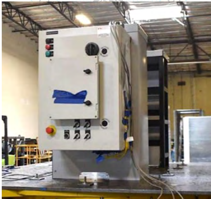
All units were filled with contents and maintained structural integrity and functionality after AC-156 test.
