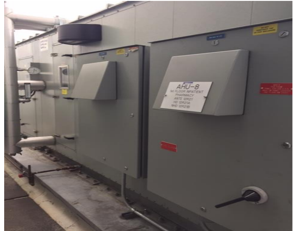
Air Handling Units and Exhaust Fans
