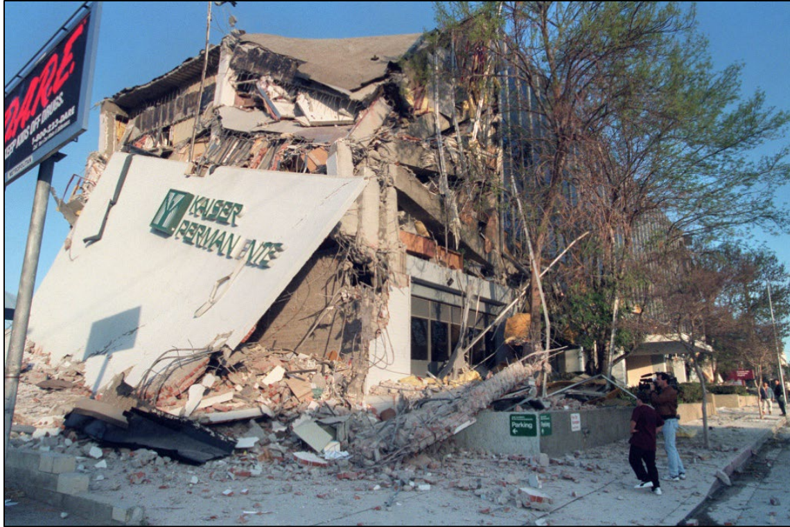
Figure 5. Damage to the Kaiser Permanente clinic building in Granada Hills during the 1994 Northridge earthquake. 5
