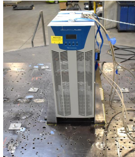
Figure 2. Front view of UUT1
