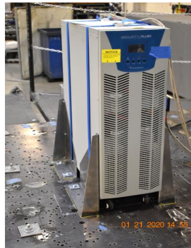
Figure 2. Front view of UUT2
