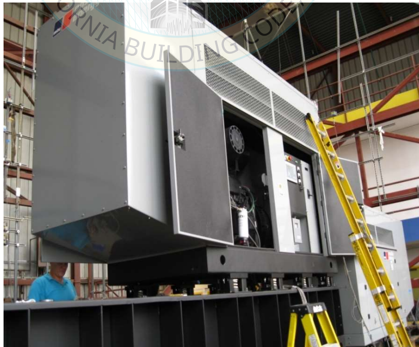
All units were filled with contents and maintained structural integrity and functionality
