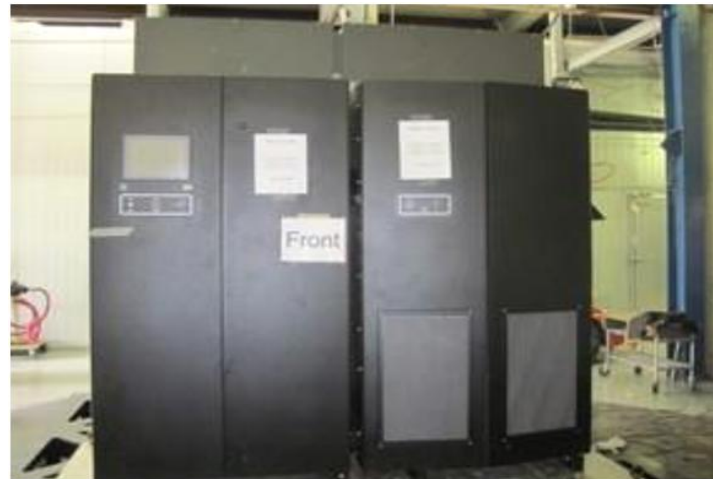
UUT #4 (Left) & UUT #5 (Right) UUT #4: Cabinet is Mounted Directly to the Table Using (4) 5/8" Diameter ASTM A490 Bolts UUT #5: Cabinet is Mounted Directly to the Table Using (6) 3/4" Diameter ASTM A490 Bolts
