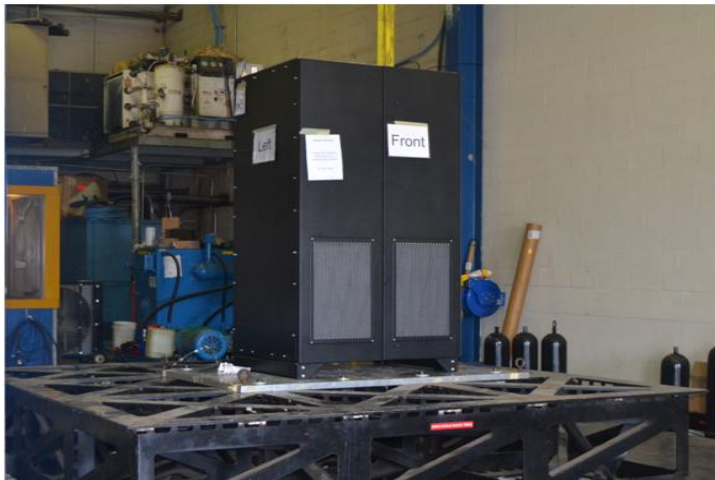
UUT #3 Cabinet is Mounted Directly to the Table Using (4) 3/4" Diameter ASTM A490 Bolts
