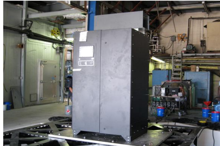
UUT #2 Cabinet is Mounted Directly to the Table Using (4) 5/8" Diameter ASTM A490 Bolts
