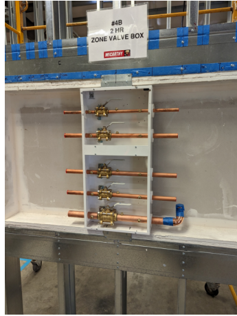
Zone Valve Box
