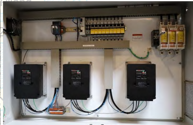
UUT-01b interior view.
