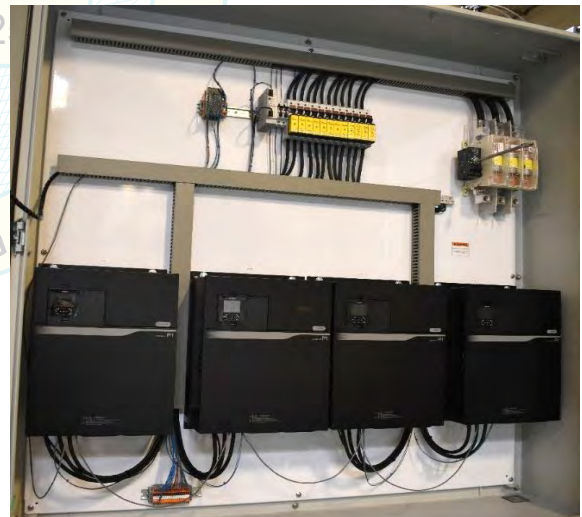
UUT-02a interior view.
