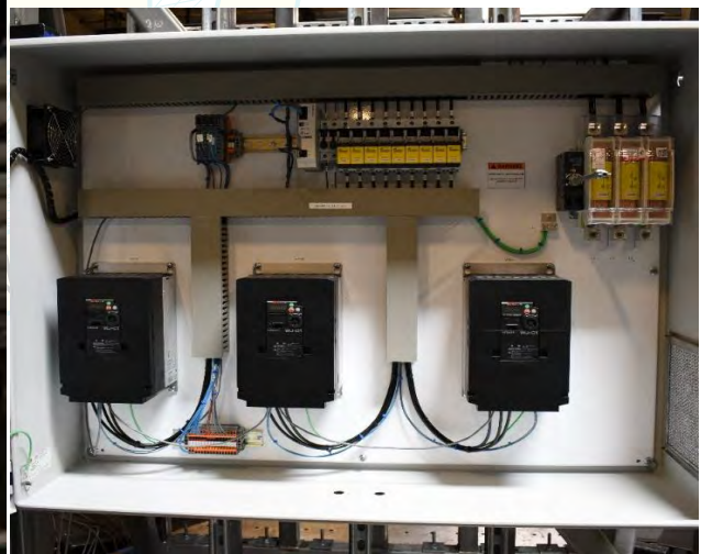
UUT-01a interior view.
