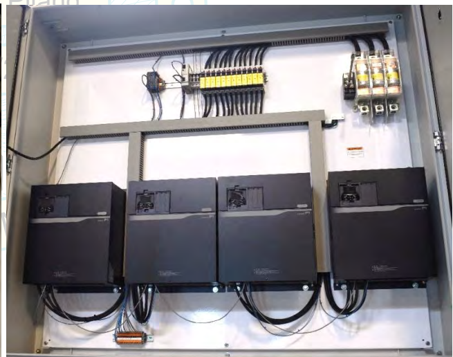
UUT-02b interior view.
